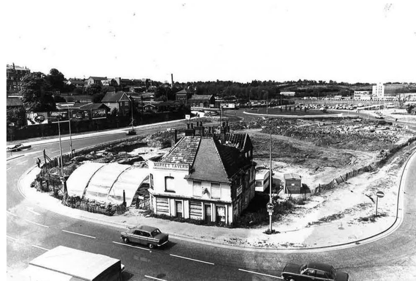
Figure 41: The site of the Cattle Market when it was cleared for the erection of the Octagon. The Market Tavern in the foreground was demolished as well.
