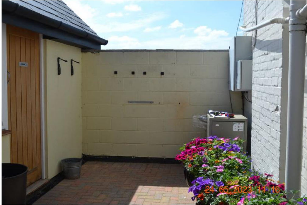
Site for new toilet as viewed from covered way to accommodation block
