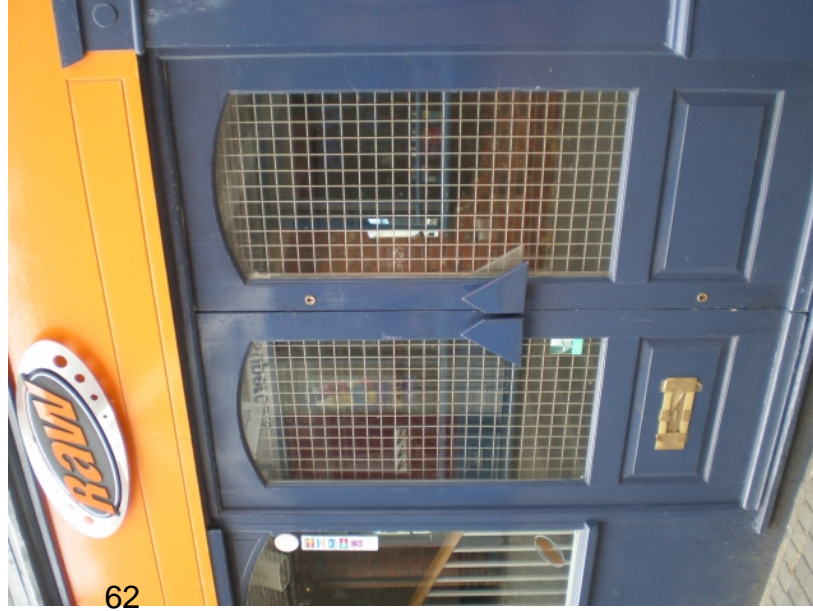
Inconspicuous internal de-mountable grille
